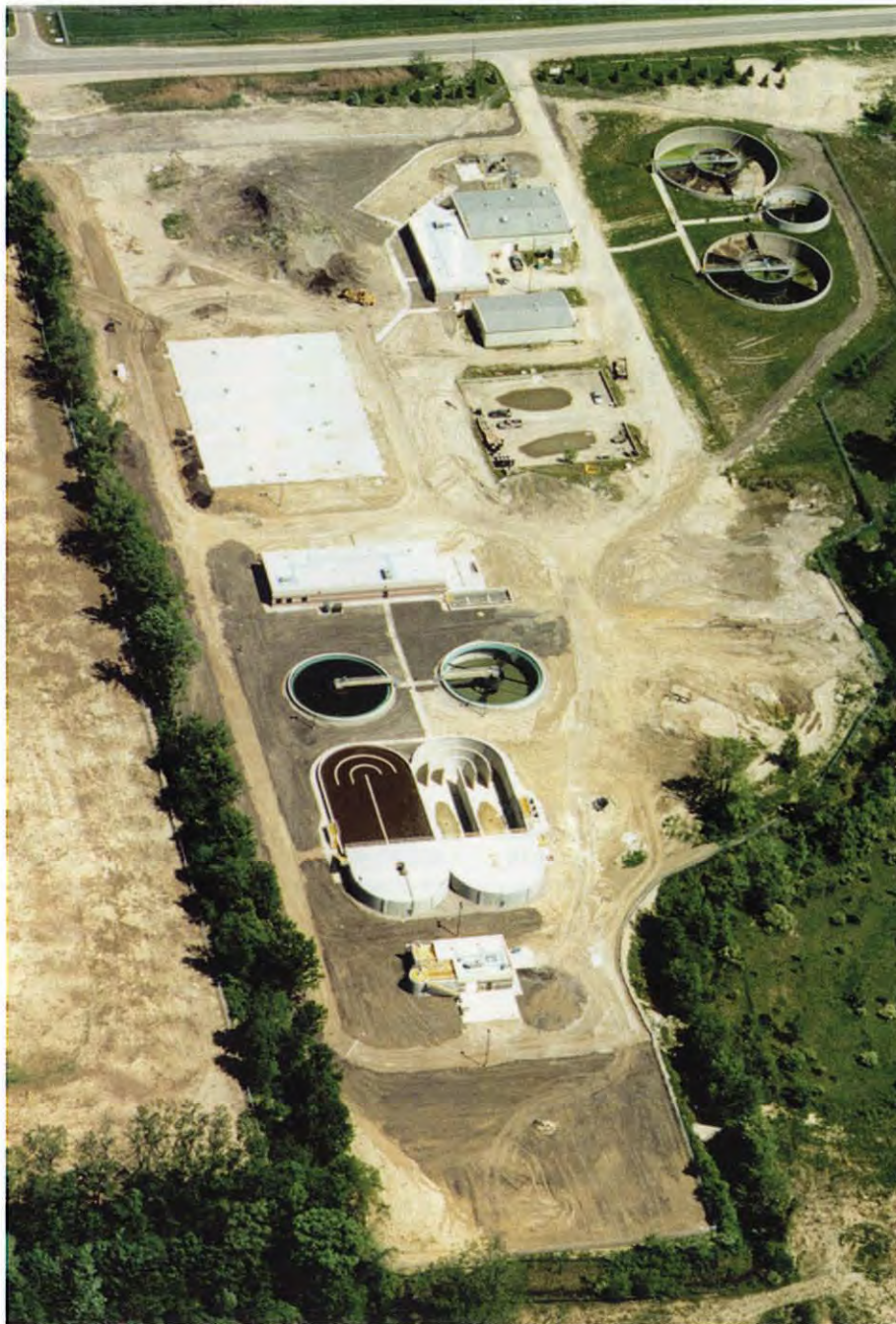
Construction of the Commerce Township Wastewater Treatment Plant is expected to be complete in early 2009. With a capacity of 8.5 million gallons per day, it will serve the needs of Commerce Township, White Lake Township, the Village of Wolverine Lake, and a portion of the City of Novi.
